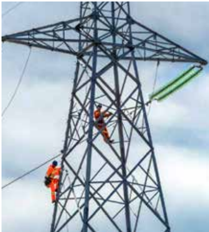
Emera Utility Services employees working on the land-based transmission for the Maritime Link in Nova Scotia.
