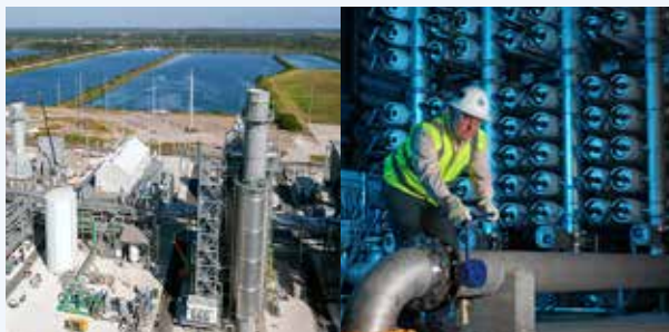
At Polk Power Station, reverse osmosis treats reclaimed water from a nearby community which is then used to cool the power station.
