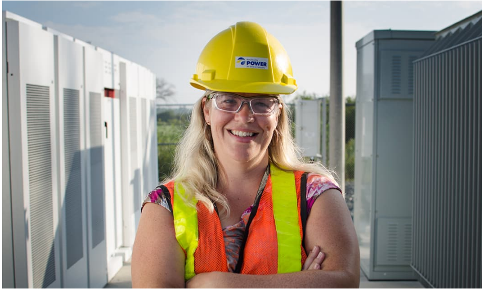
A Nova Scotia Power employee at the Intelligent Feeder Project in Elmsdale, Nova Scotia. This pilot project is helping us understand how new technology can improve service for customers.
