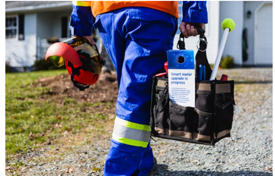
Our teams are working hard to install smart meters for customers across our electric utilities. This technology will provide customers with more information about their energy use and allow utilities to identify and respond to outages more efficiently.
