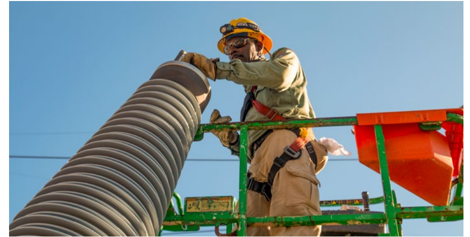
Safety is top of mind for this member of the Tampa Electric team who is working on the modernization project at our Big Bend facility.
