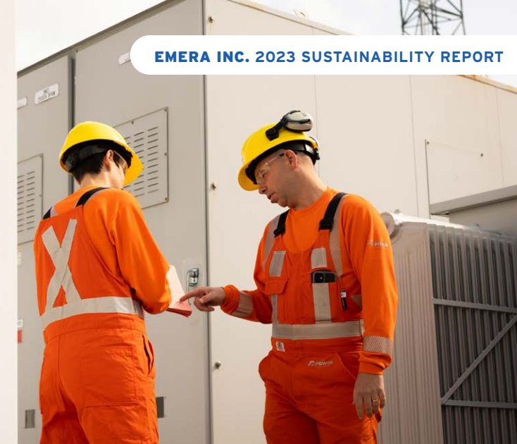
Nova Scotia Power team members at the Intelligent Feeder Battery Storage Pilot in Elmsdale, NS.
